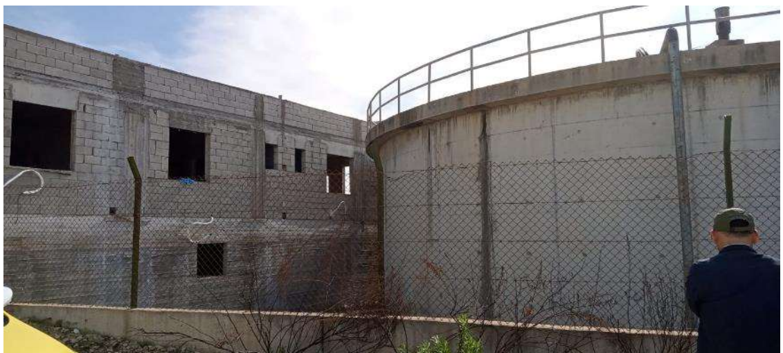
Photo for Land of Burqin Booster Pumping Station within Al-Jabriyat Tank Site
